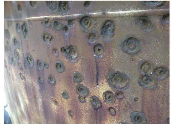
Exterior corrosion on uncoated silo
